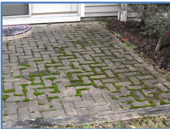
Moss Growth Between Pavers
