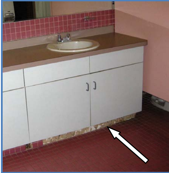
Missing Tile – Women's Room Vanity
