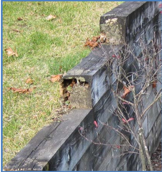
Deteriorated Top Retaining Wall Rail
