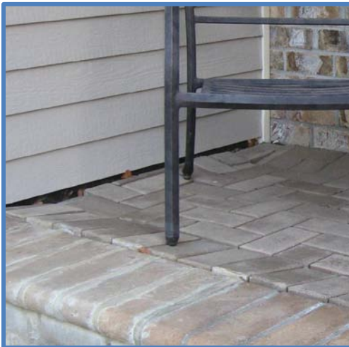
Sunken Pavers at Front Porch
