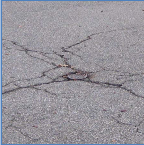
Pavement Failure at Water Valve
